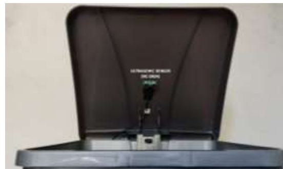
Figure 20. Front View of the Inside of the Node Device
