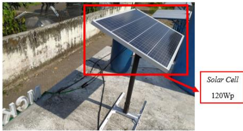
Fig. 14. Solar cell on top of public toilet
