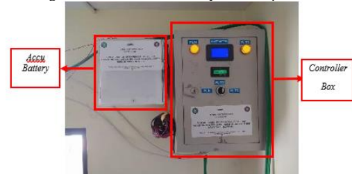
Fig. 13. Solar cell Hybrid System Power Management Hardware
