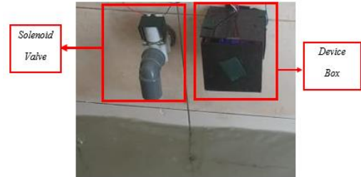
Fig. 10. Public Toilet Water Tank Filling Hardware
