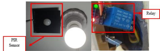
Fig. 12. PIR Sensor and Relay For Lamp Control
